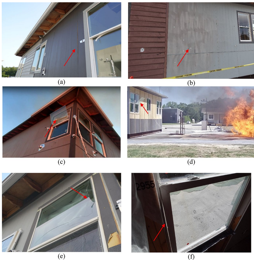
Fig. 5 Example of Envelope damage: a fiber cement siding bowing and (b) cracking; window damage including (c and d) pane detachment, e glass fracture, and f sash deformation
