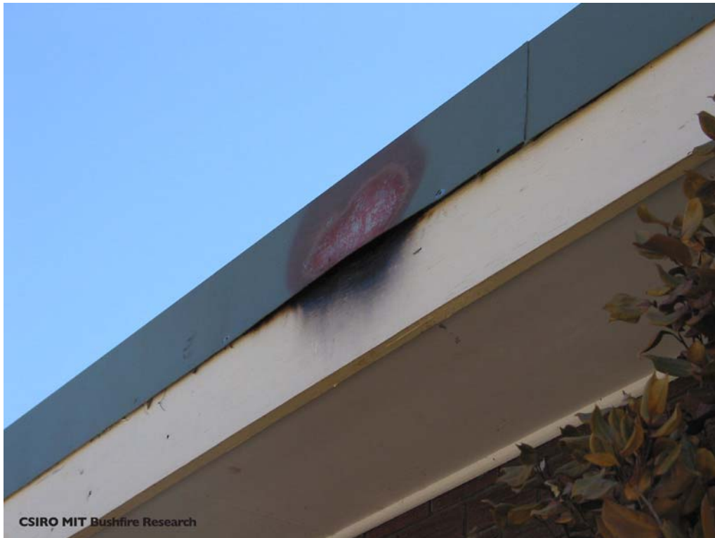
Figure 35. Ember attack on poor fitting capping
