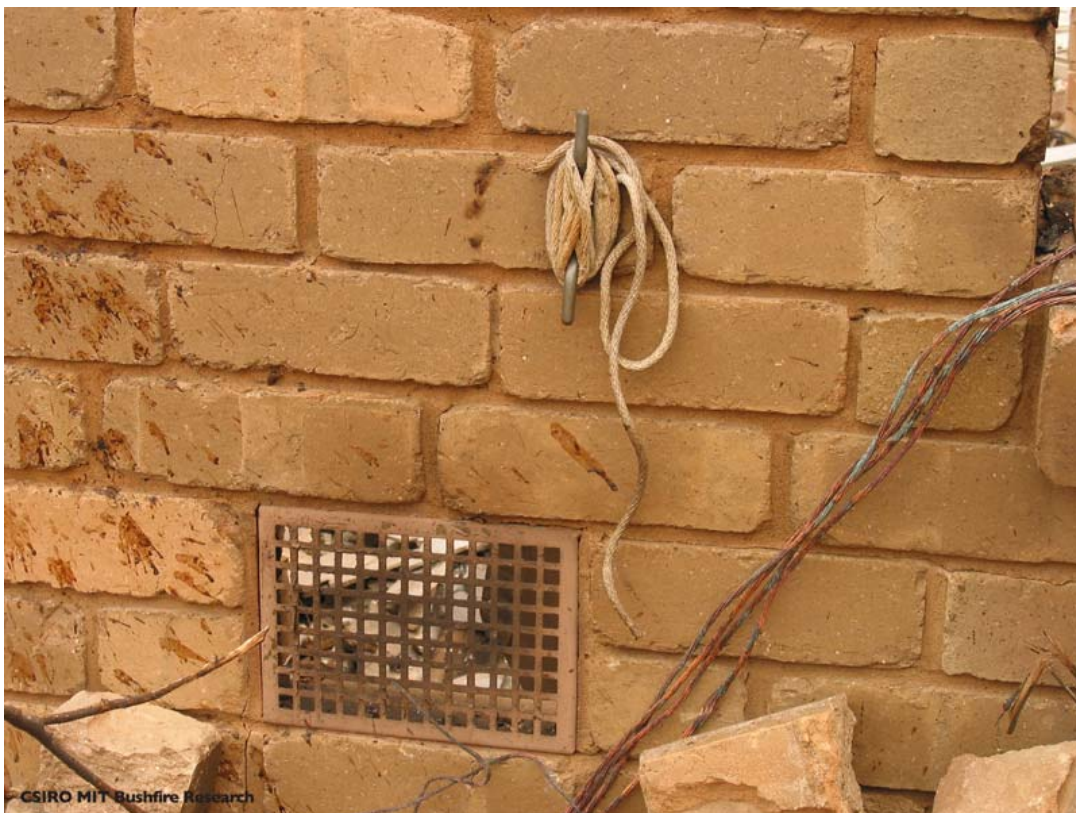
Figure 31. Typical unprotected vent
