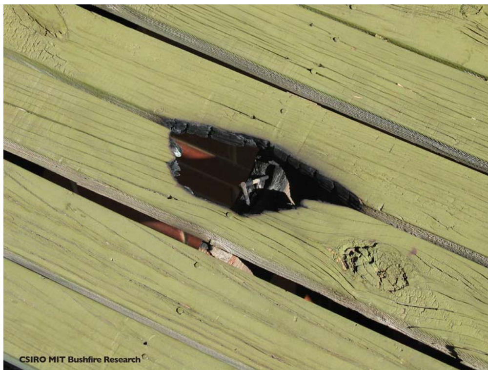
Figure 38. Ember attack on deck (with intervention)
