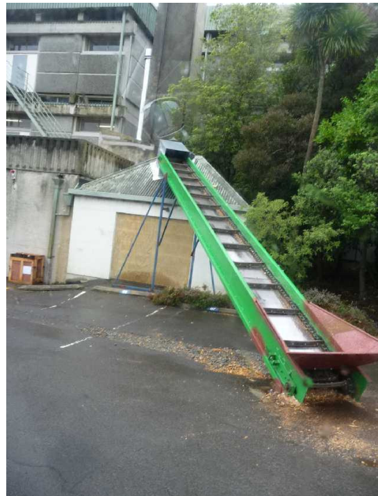
temporary storage and inclined chip transfer system for Otago University 1100 kW Binder boiler
