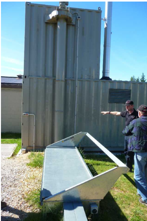
Wanaka pool above-ground chip transfer auger to storage and 110 kW boiler in container
