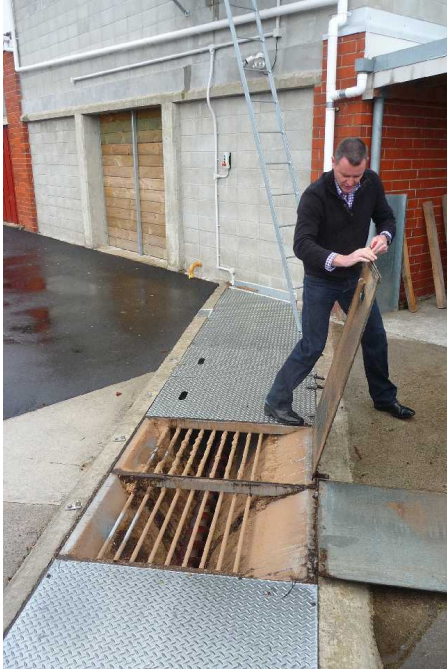
Inground chip transfer auger to vertical auger within storage immediately behind (see to right)
